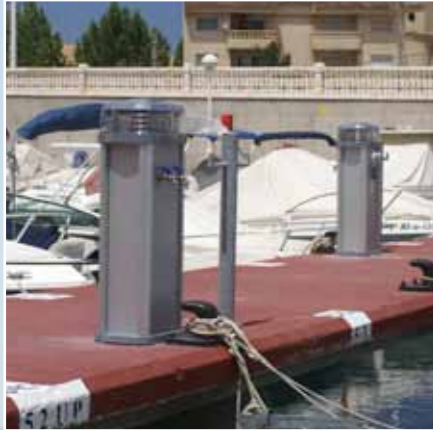
Electricity and Water Pedestals
